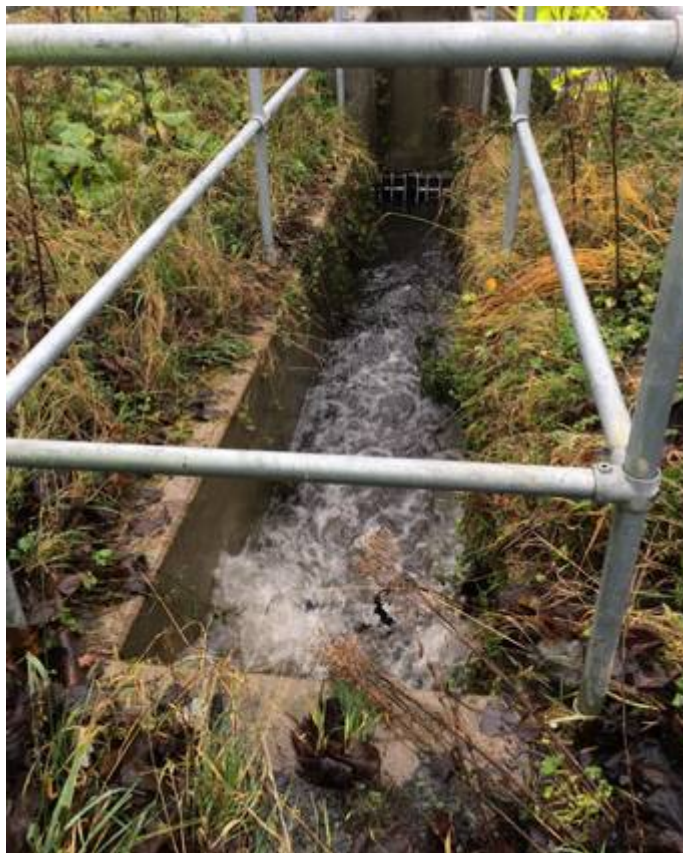
Figure 5 : reduced water level at culvert by approx. 500mm following removal of blockage to the trash screen
