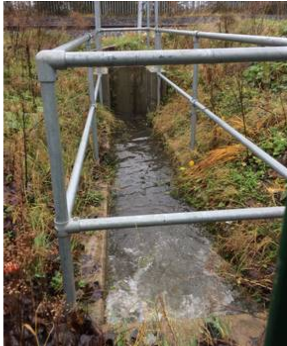
Figure 4 : raised water level at culvert entrance due to debris blocking the trash screen at the entrance to the culvert located in Irish Rail Property
